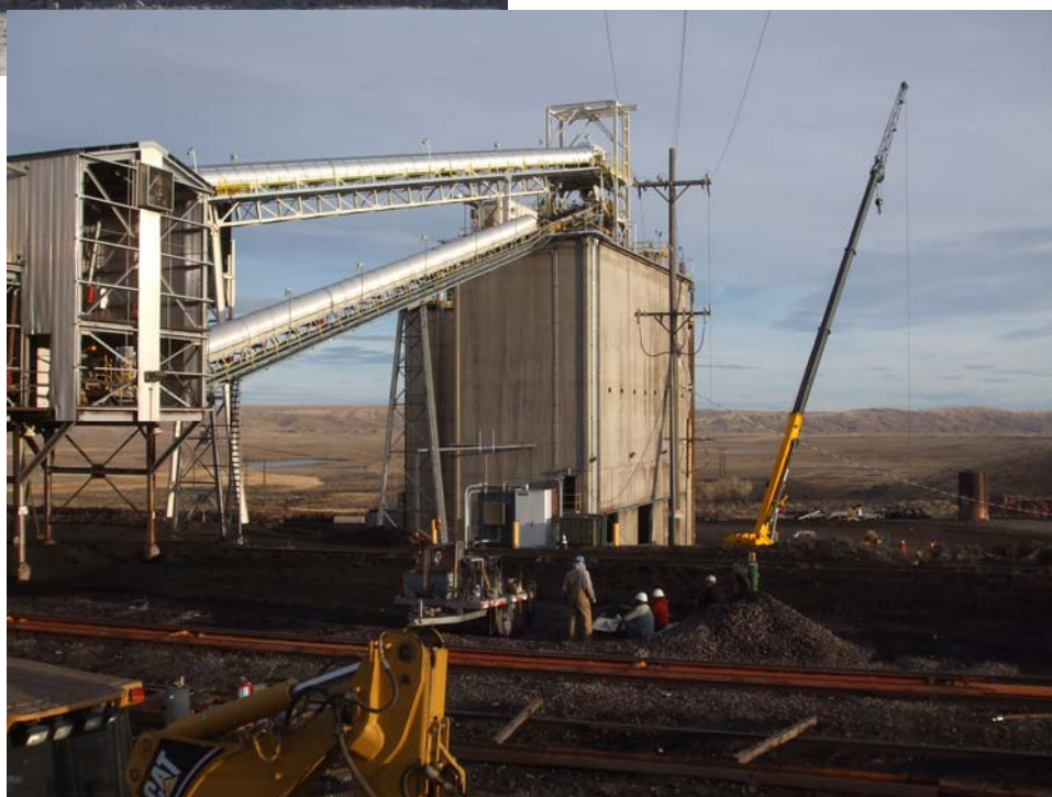
Truck loadout feed conveyors CV-450 (top) existing conveyor (bottom)
